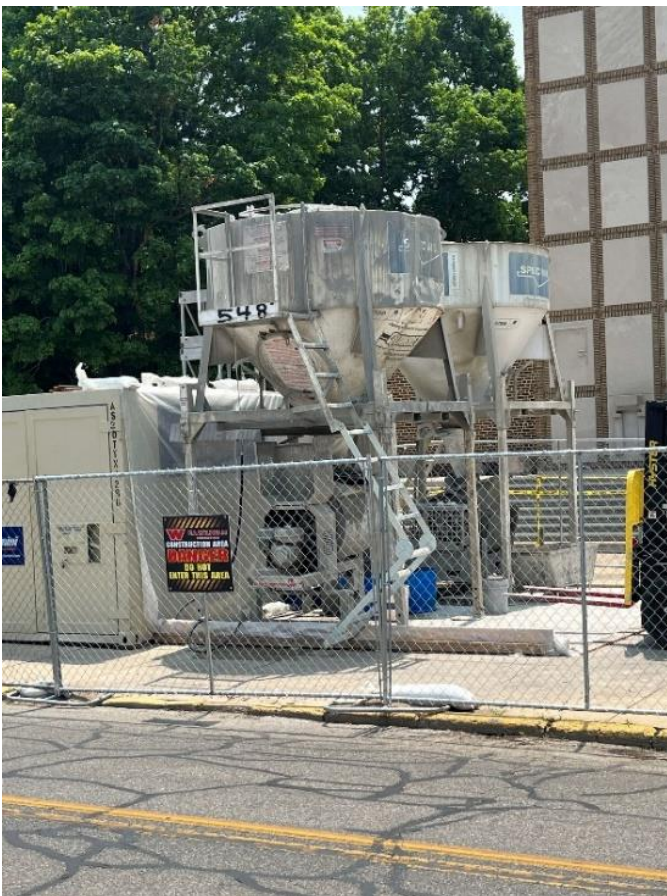
Large batch mixers were set up to allow for blending cement, sand, and water creating the necessary mortar in both strength and color for brick replacement and tuck pointing.
