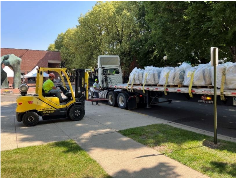
A truckload of dry premixed cement and aggregate was received and unloaded for use. Obtaining it this way allowed for better quality control and color consistency.
